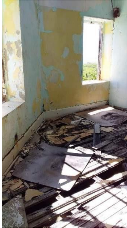
Figure 123. Accessory structures at Hole in the Wall Lighthouse in disrepair.
