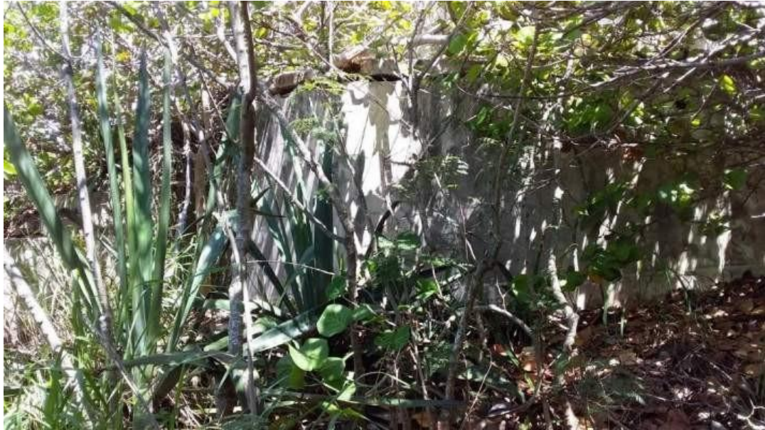
Accessory structures at Hole in the Wall Lighthouse in disrepair.
