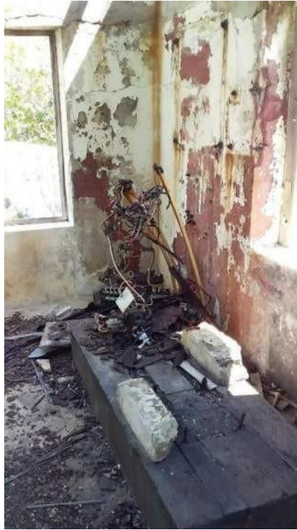
Figure 122. Accessory structures at Hole in the Wall Lighthouse in disrepair.
