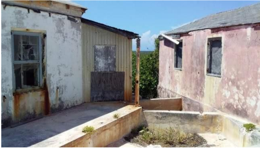
Figure 118. Accessory structures at Hole in the Wall Lighthouse in disrepair.
