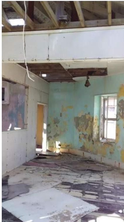
Figure 124. Accessory structures at Hole in the Wall Lighthouse in disrepair.
