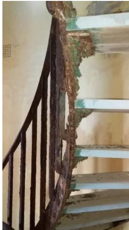
Figure 116. Stair supports in Hole in the Wall Lighthouse showing signs of rust.
