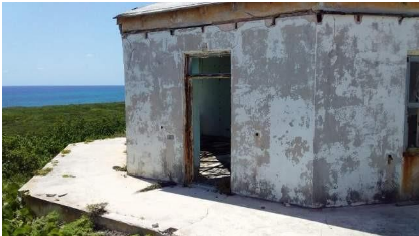
Figure 119. Accessory structures at Hole in the Wall Lighthouse in disrepair.
