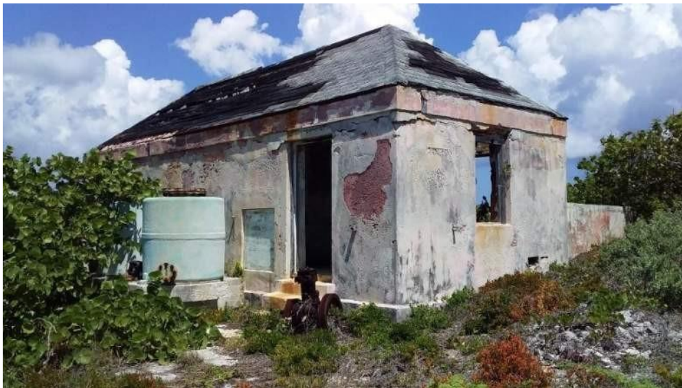
Figure 117. Accessory structures at Hole in the Wall Lighthouse in disrepair.
